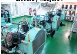
Compressors / Chillers / Reefers :
